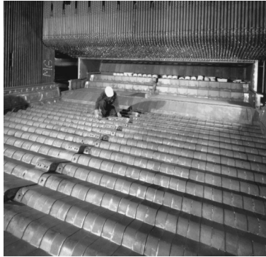
Figure 1.5: A picture of a new horizontal forward acting grate. The waste enters at the back of the picture and travels towards the viewer. The boiler tubes at the furnace walls can be seen as well. Source: Martin GmbH für Umwelt- und Energietechnik
